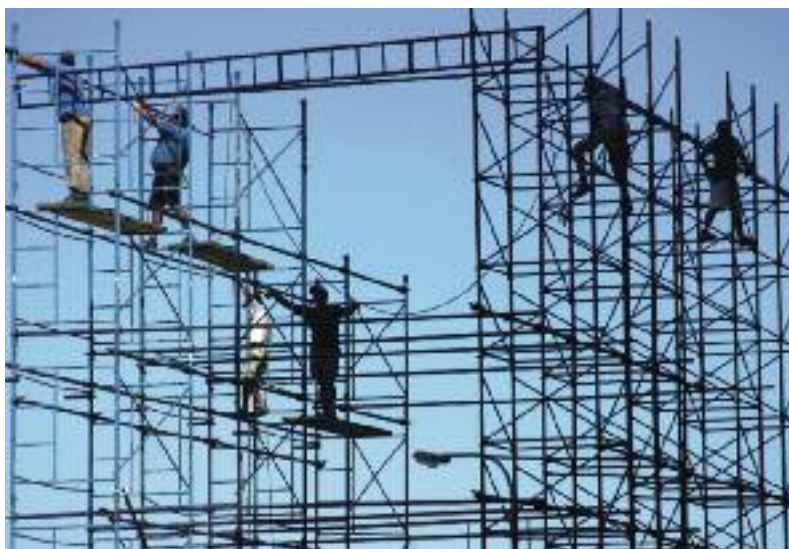
Dangerous construction site. Author: Peter Rimmer
